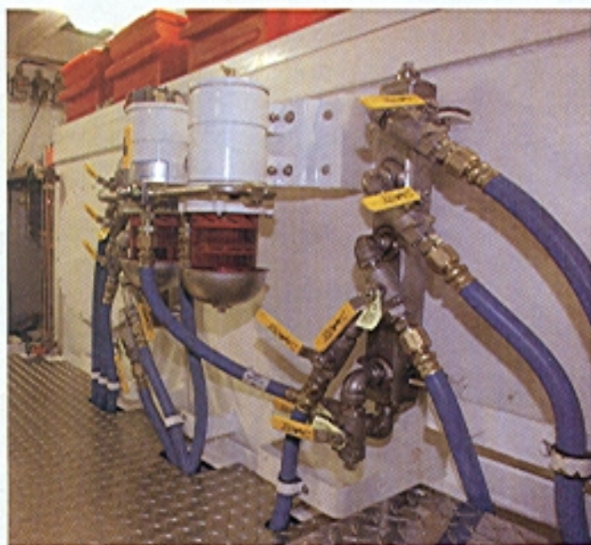
The easy-to-access fuel filtering system includes proper filters and fire-rated hoses and makes filter changes easy.
