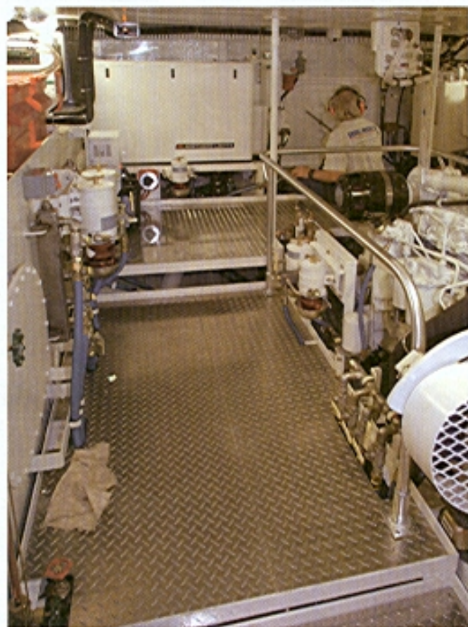
The engine room of the Neville 47 is a good example of proper engineering, with easy access to systems and machinery. This view is looking aft through the access hatch.
